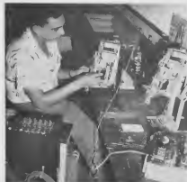
AN ELECTRICAL operation of an exchange selector is inspected by C. Pierre so that maximum efficiency of telephone exchange equipment is maintained.
